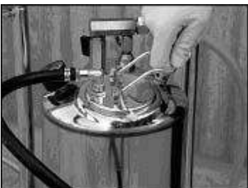
Open fastener on pressure vessel.
